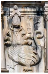
fig.49 Details of the stone facade Ruins of St. Paul, built from 1582-1602, Macau
